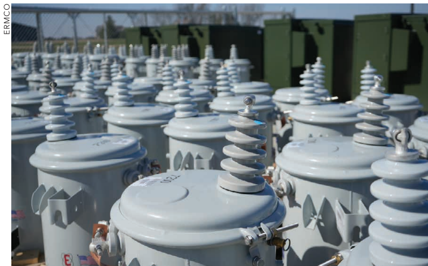
SHORT SUPPLY: Electric co-ops are seeing lag times of up to four years between orders for transformers and their delivery. The price has also doubled since the COVID-19 pandemic.
