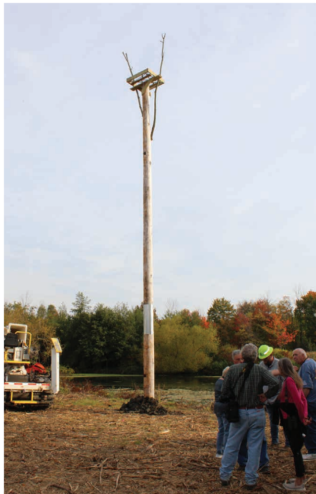
COMMUNITY EVENT: Friends, family and community supporters gather to see the osprey structure at Peninsula Park. Northwestern Rural Electric Cooperative crews raised the structure, designed by Eagle Scout candidate Ethan Snyder of Edinboro.
